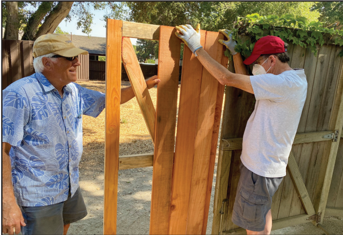
Dave Backs and Harry Guy installing new extension "wings" on the back gate.
